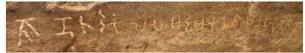
Fig. 2. A representative Brahmi inscription from the Anuradhapura archaeological zone, showing typical surface degradation, weathering, and character erosion.
